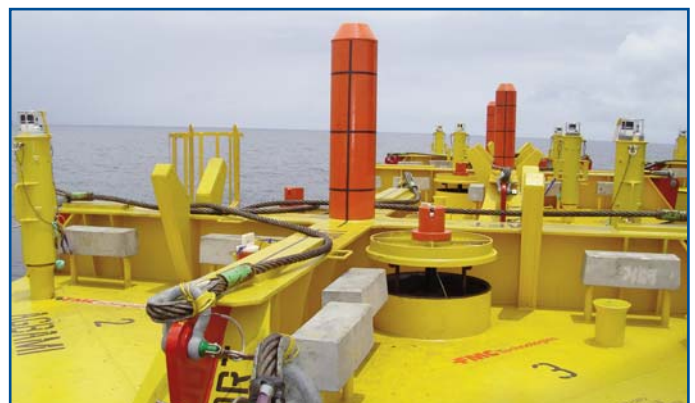
NASNet® MTrx mounted on suction piles
